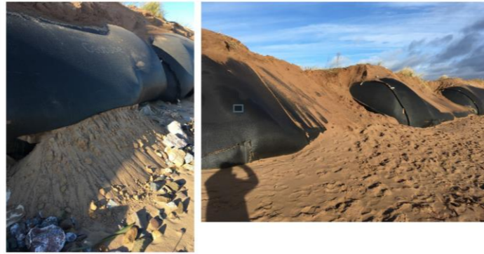
Geotube vandalism & damage
