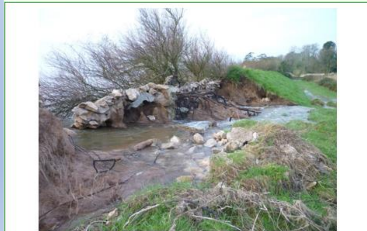
Figure 4: Photo of 2014 Breach of flood bank
